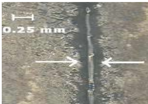
Fig. 4: Crack repaired with epoxy
