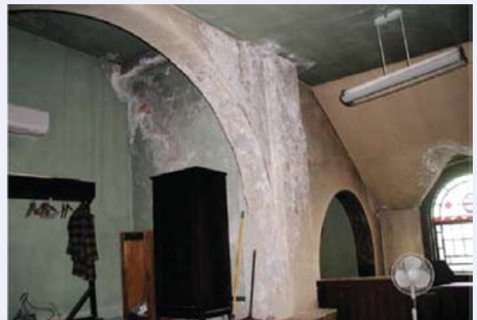
Fig 3: Distress in internal walls
