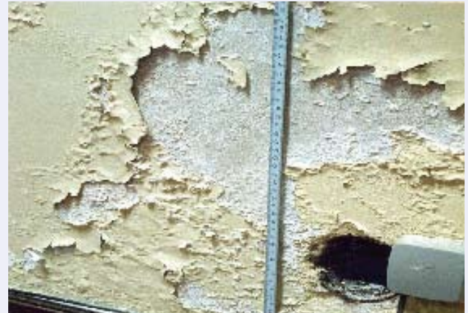
Fig: 2 Salt damage of weak pointing material
