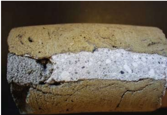
Fig: 4 Dense repointing leading to frost damage
