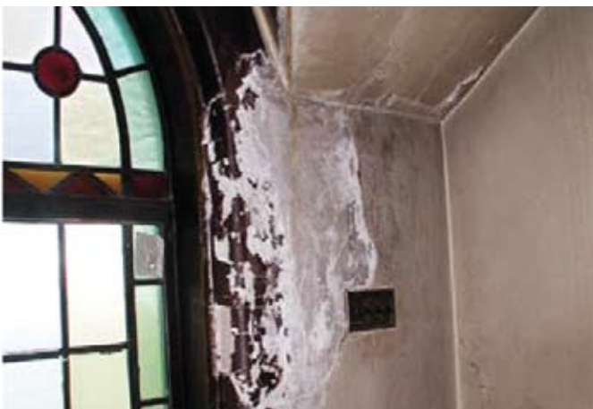
Fig 2: Distress in plastering
