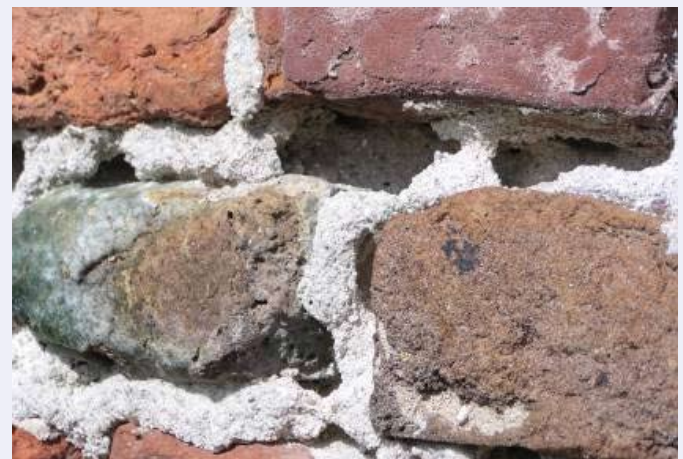
Fig: 3 Damage through salt Crystallization
