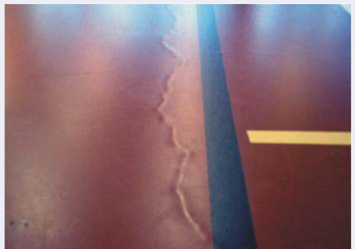
Fig. 9: Extrusion of crack filler beneath poured polyurethane gymnasium flooring
