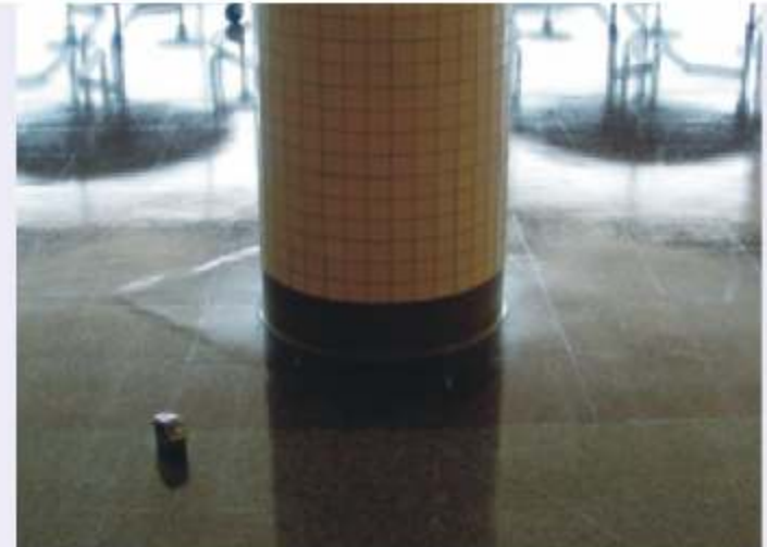
Fig. 5: Reverse wrapping around isolated diamond blackout at column footing
