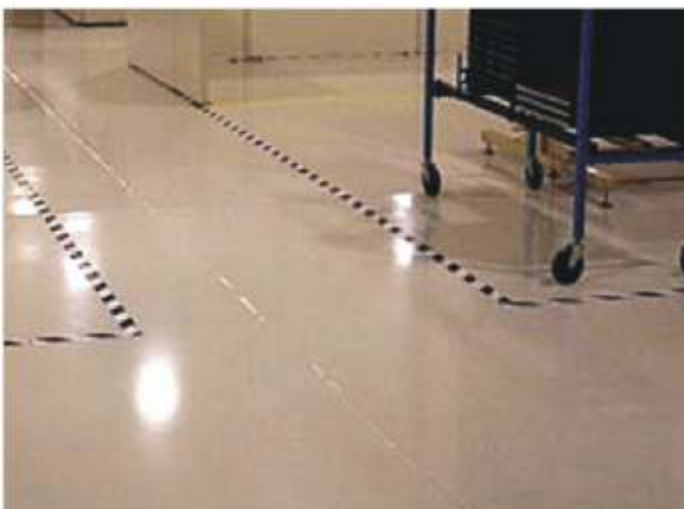
Fig. 2: Extrusion of semi-rigid joint filler due to reverse warping (photo courtesy of Herman Prozel)
