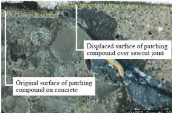
Fig. 4: Photomicrograph in reflected light showing details of patching compound movement upward. Dotted line indicated original surface and displaced surface due to movement. The black gap at top left is the space created when tile was pulled loose from the patching compound, forming a bubble
