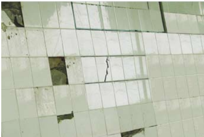
Fig 2 : Failure due to thermal movement
