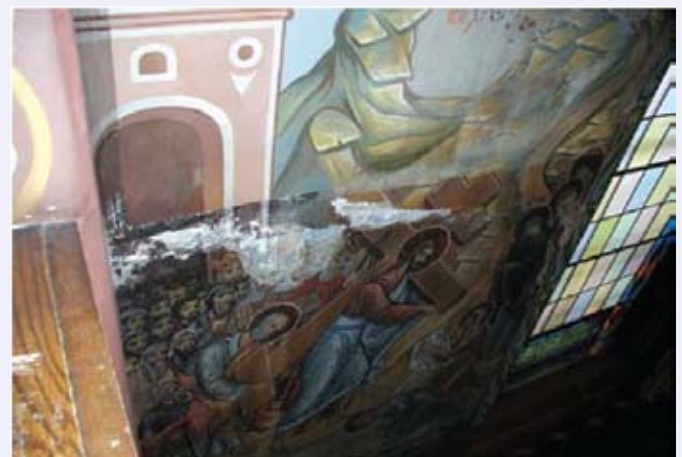
Fig 4: Damages in wall paintings
