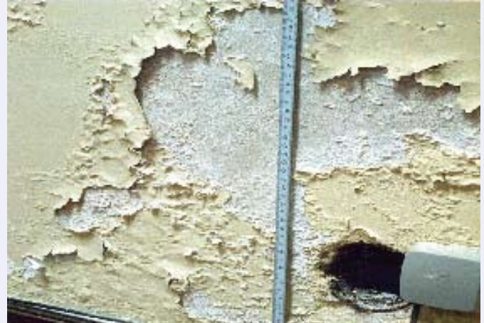
Fig: 2 Salt damage of weak pointing material
