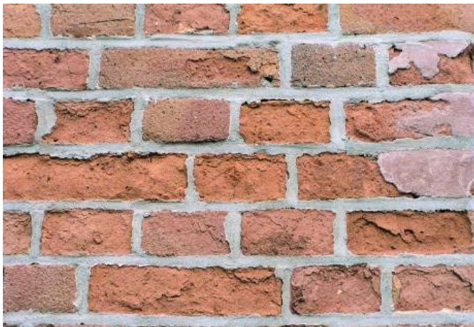
Fig: 5 Subflorescence caused by water repellents
