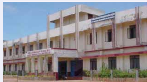
Fig. 13: Before repair in distress conditions
