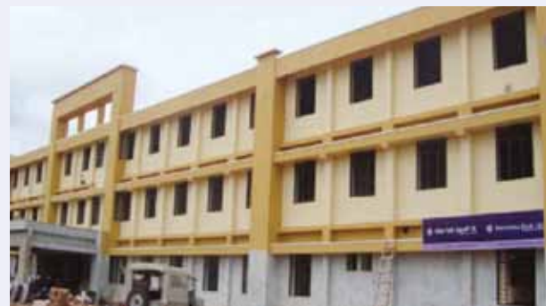
Fig. 14: View of the same building after repair, strengthening and with an additional floor
