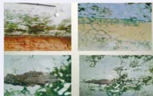
Fig. 4: Fungal growth on ceiling
