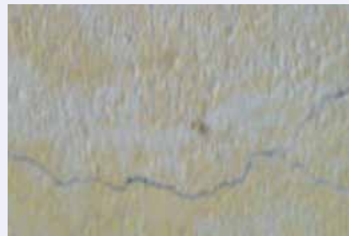
Fig. 3: Cracks in the ceiling
