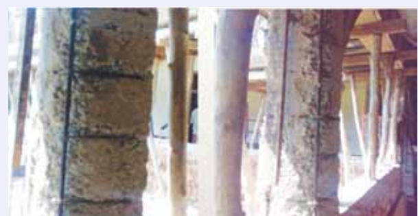
Fig. 5: Corrosion of reinforcement and spalling of concrete in columns
