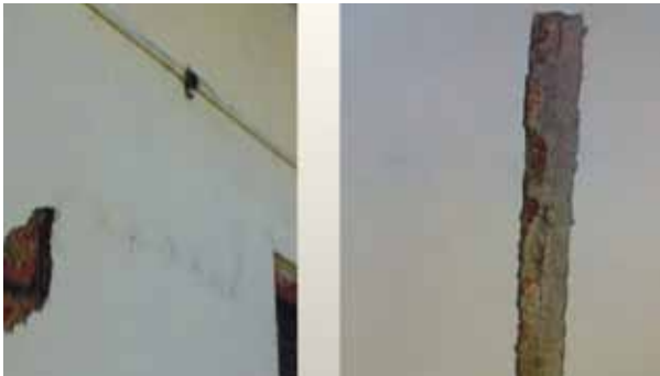
Fig. 6: Cracks in walls
