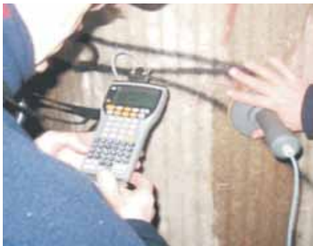
Fig. 3: Corrosion monitoring of a heavily corroded column
