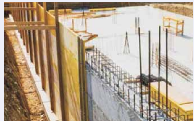
Fig. 9: SBS sheet membrane applied in double layer to concrete foundation wall in a basement
