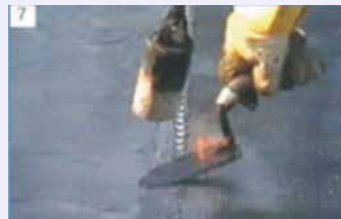
g. Heat both the overlaps & use round tipped trowel to seal overlap
