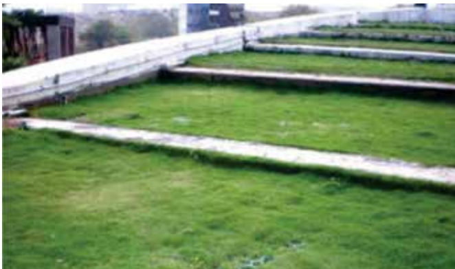
Fig. 5: Above figure reveals a section of structural pavers where the sod is thinned, likely a seam
