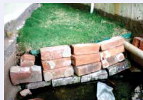
Fig. 7: Being the first of its kind on the subcontinent, the green roof's drainage system is exemplary of pioneering resolve and locally-inspired innovation.
