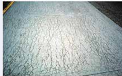
Fig. 2: Longitudinal cracks induced by ASR in a pavement
