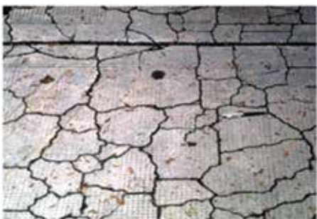
Fig. 11: Map cracking pattern caused by ACR
