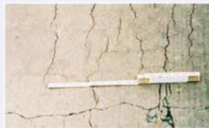
Fig. 3: Close-up view of well developed cracking in a pavement, a typical pattern associated with ASR.
