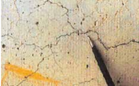
Fig. 4: Map pattern cracking due to ASR
