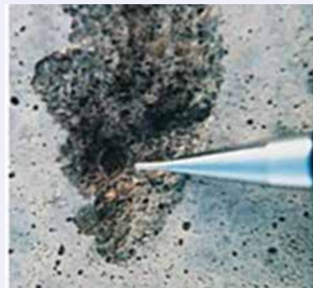
Fig. 6: Popouts due to ASR
