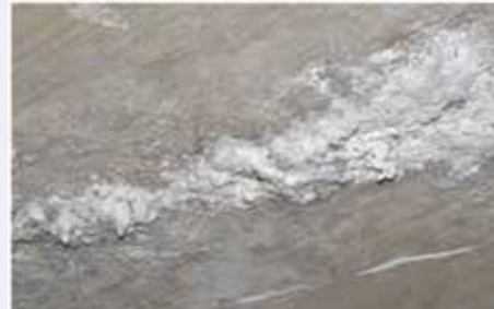
Fig. 5: Efflorescence due to ASR patterns
