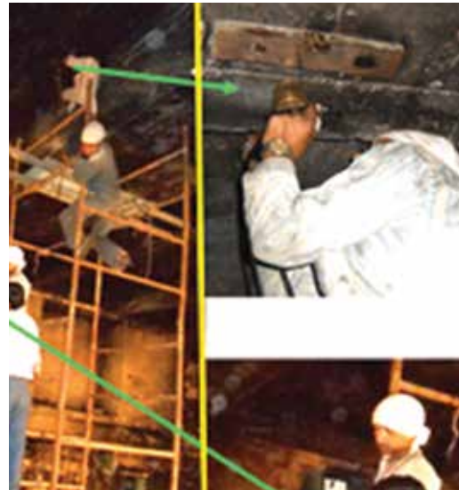
Fire damage assessment of an auditorium building
