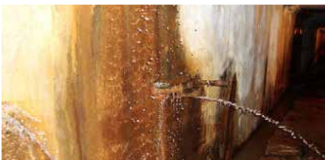
Fig. 2 : Water leakages in the drainage gallery.
