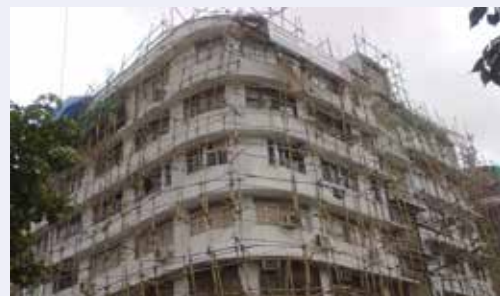
Fig. 8: View before repair
