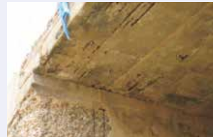
Fig. 3: Spalled concrete in the piers
