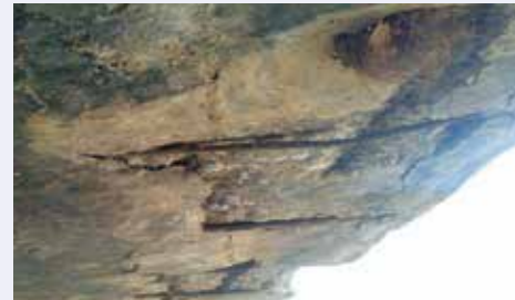
Fig. 1: Spalled concrete at the edges
