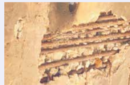
Fig. 2: Spalled concrete and reinforcement corrosion
