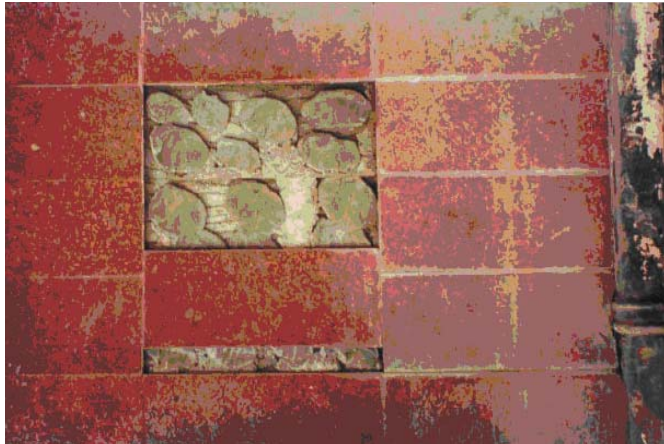
Fig 1 : Adhesion failure due to use of cement as adhesive
