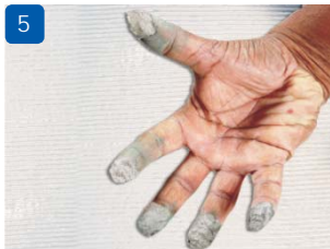
5 Touch the paste intermittently and if sticks to finger then continue tiling
