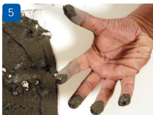
5 Touch the paste intermittently and if it sticks to finger then continue tiling
