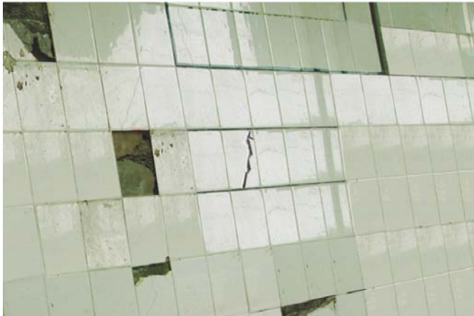
Fig 2 : Failure due to thermal movement
