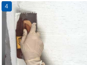
4 Apply the adhesive paste on a tiling substrate with 2 mm notch trowel
